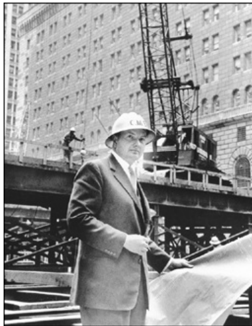
The construction of Chase's new headquarters in the early 1960s. Our building was the first step in the revival and redevelopment of Wall Street. (Courtesy of the J.P. Morgan Chase & Co. Archives)
